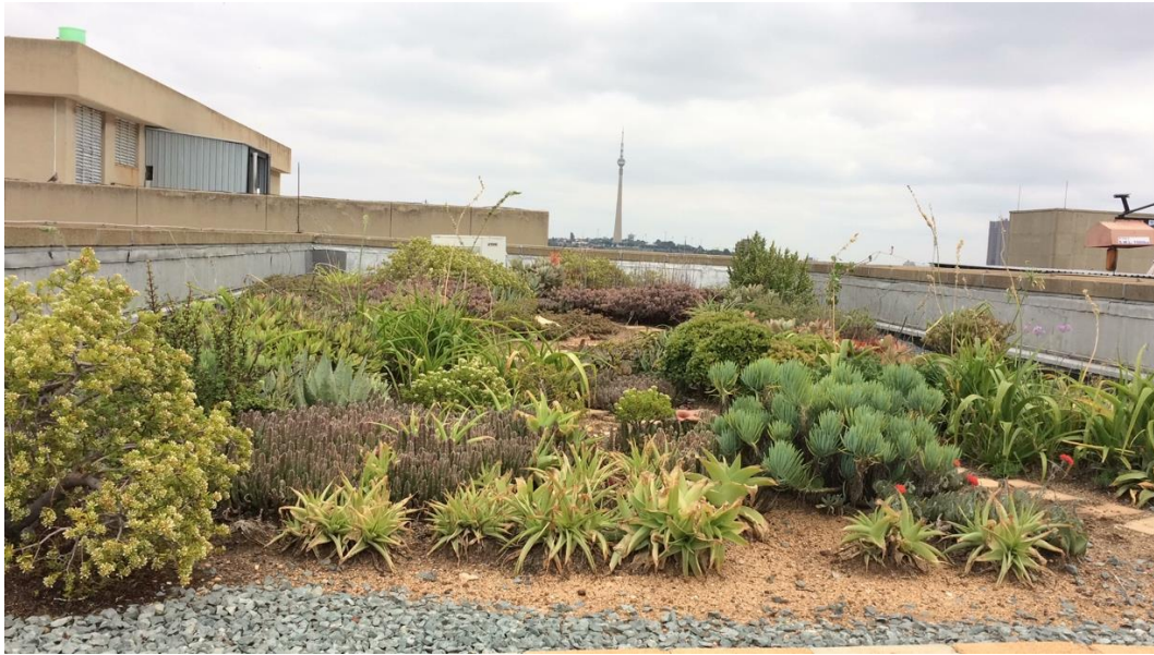
Figure C1: Extensive green roof at University of the Witwatersrand
